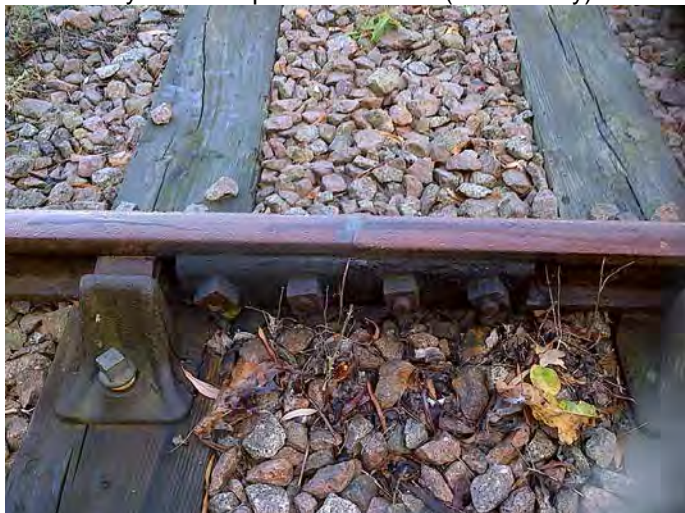
D5 - Catchpit found at 693.2m (91M 1705y)
