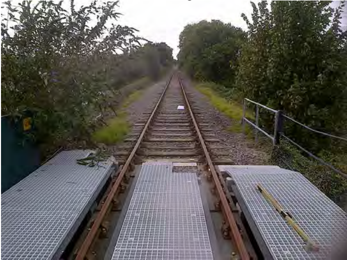
D28B - Longitudinal timber bridge 6249m 6260.2m back to high mileage (95M 748y – 95M 761y)
