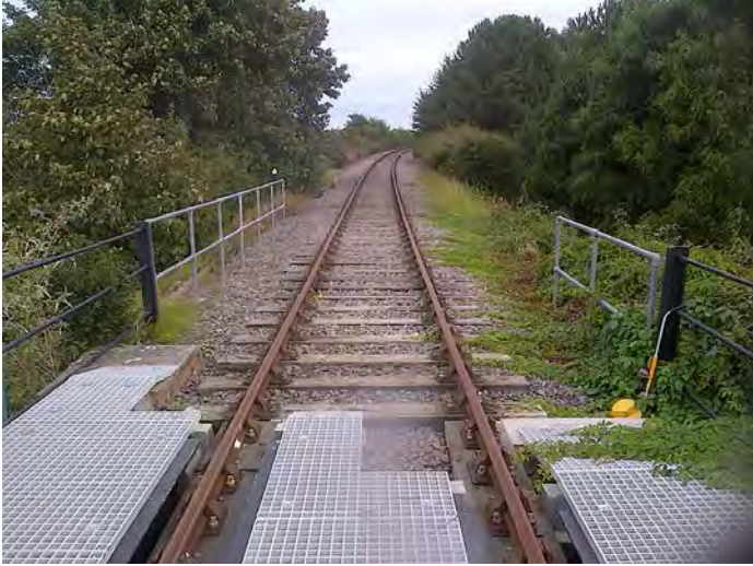
D28C - Longitudinal timber bridge 6249m 6260.2m back to low mileage (95M 748y – 95M 761y)
