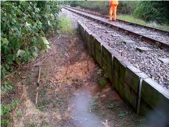
D30 - Embankment burrowing issue 6286.1m (95M 789y)
