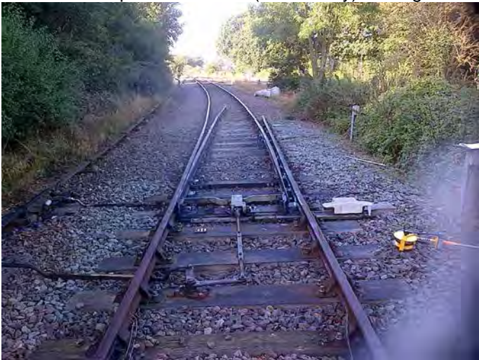
D3 - 3B catch points at 75.8m (91M 1028y) looking towards low mileage
