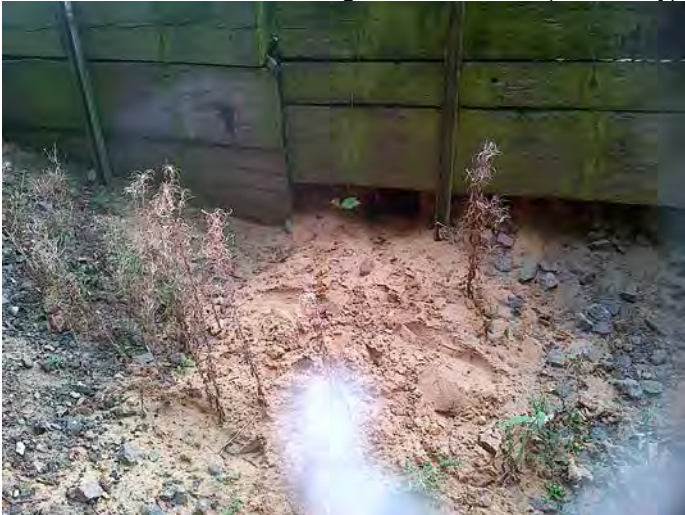
D29 - Embankment burrowing issue 6286.1m (95M 789y)
